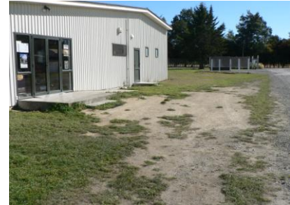
Example area requiring maintenance due to high traffic use (Issue: dust and drainage)
