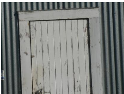
Example maintenance required (Issue: paint deteriorated)
